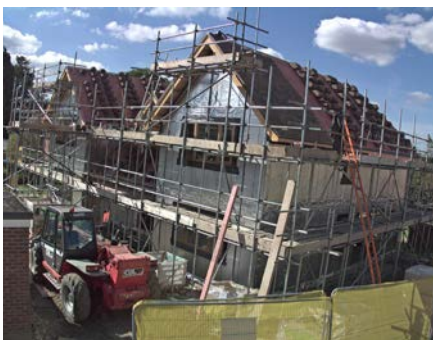
On completion of the shell, work on the roof tiling can commence.
