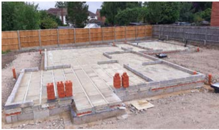
The foundations are prepared ready to receive the timber frame from the factory.
