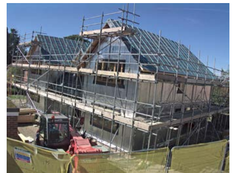
The roof is fully boarded, felted and counter battened by the shell erectors.
